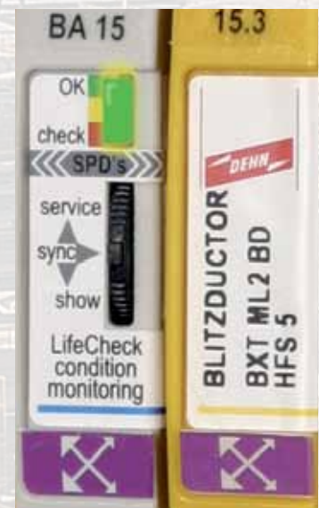
DRC MCM XT monitoring device with visual status indication installed next to a BLITZDUCTOR® XT with LifeCheck®
